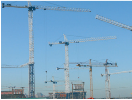
▲ Large construction site with multiple crane use. Anti-collision systems help to prevent accidents.
